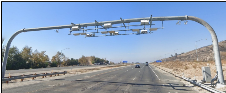
Figure F1 - Overhead gantry with vehicle sensors on SR-241. Source: Google Maps.
