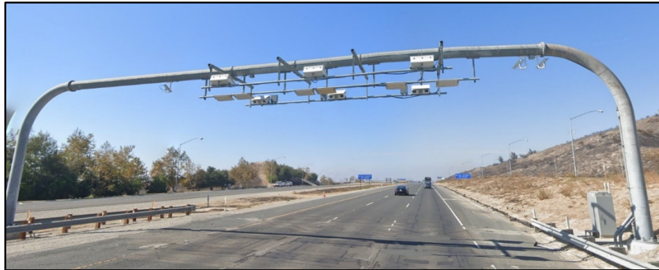
Figure F1 - Overhead gantry with vehicle sensors on SR-241. Source: Google Maps.
