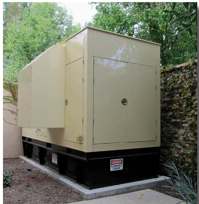
Emergency electrical power generator available to power an EOC during electrical outages.
