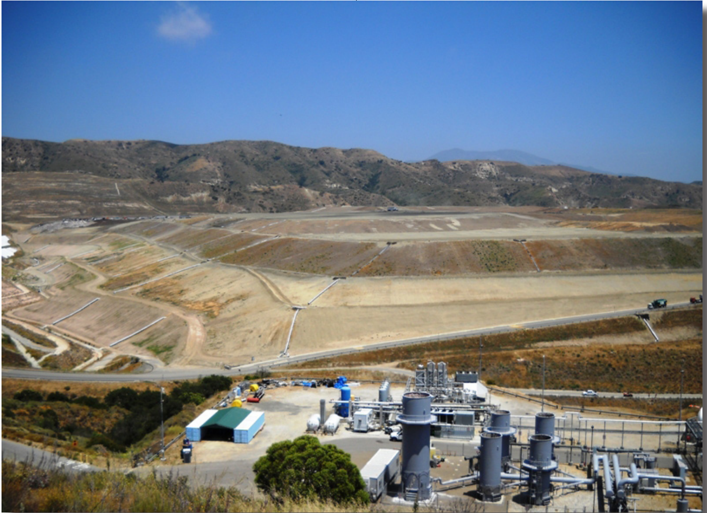
Methane gas conversion to LNG plant located at Frank R. Bowerman Landfill.
