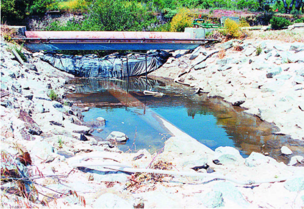
J03P02 Storm Drain outlet to Aliso Creek
