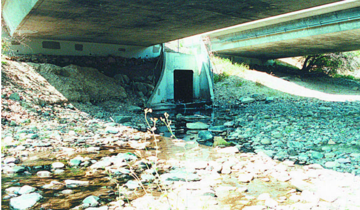
Munger Storm Drain in Upper Aliso Creek Watershed
